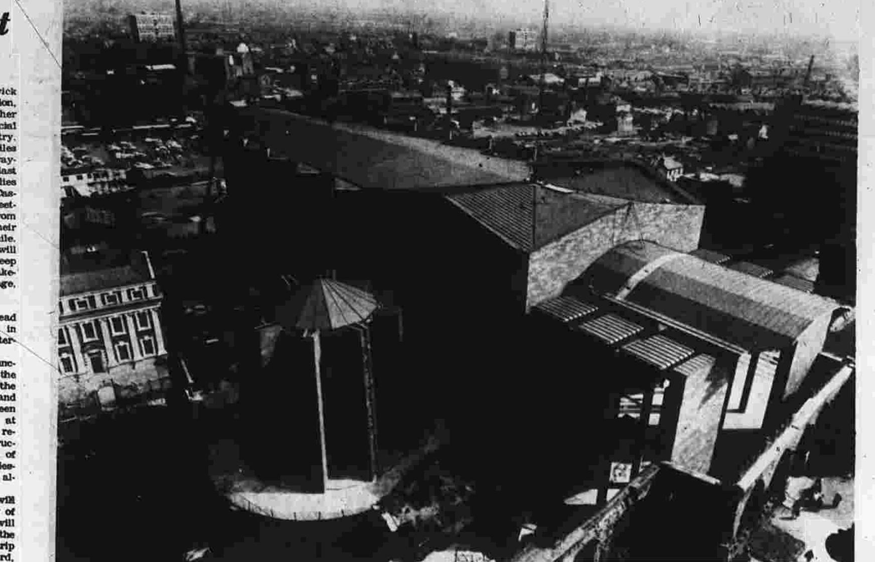
New Coventry Cathedral going up 25 years ago. Walls of old one, hit by Nazis, are in foreground. At left, Chapel of Unity.
